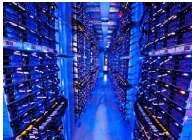
Microsoft's Chicago datacenter
