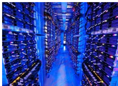
Microsoft's Chicago datacenter
